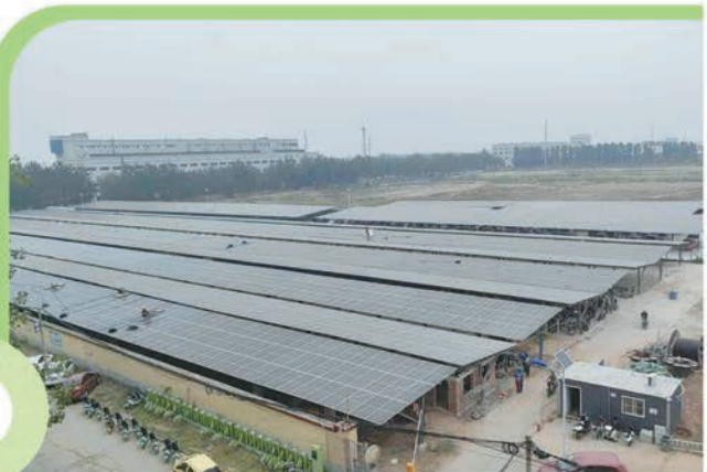
Leased photovoltaic power generation equipment 光伏電力生產租賃設備
