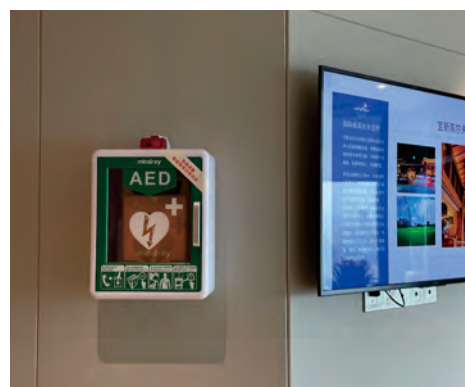
AED equipment in office area 辦公區域AED設備
