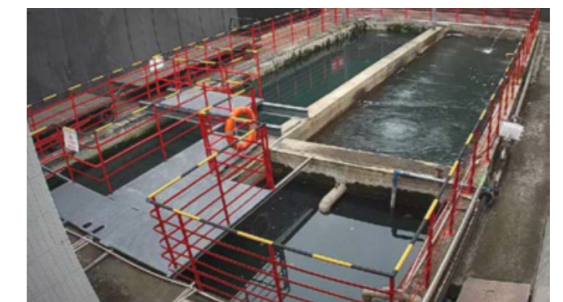
COFCO Coca-Cola Sichuan plant wastewater treatment facility 中糧可口可樂四川廠廢水處理設施
