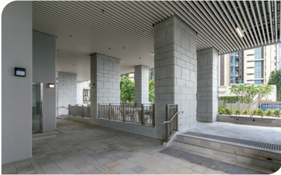
Construction of public housing development at Java Road, North Point – Design, supply and installation of suspended ceiling system at podium level 興建北角渣華道之公共房屋發展項目－設計、供應及安裝平台層之假天花系統
