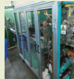
Frame safety door 框架安全門
