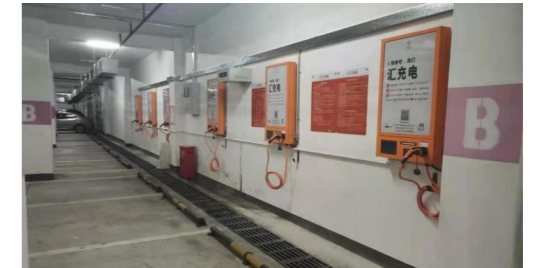
Electric vehicle charging stations in the basement carpark of Technology Building 科技大廈於地庫停車場的電動車充電站
