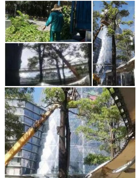
Typhoon-proof reinforcement works in Garden City Shopping Centre 花園城的防颱風加固工程
