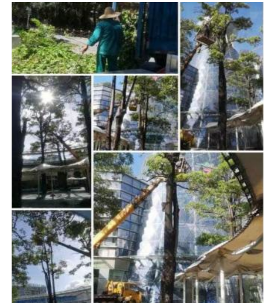
Typhoon-proof reinforcement works in Garden City Shopping Centre 花園城的防颱風加固工程
