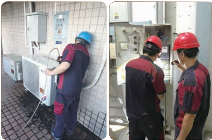
Regular Maintenance of Property Facilities and Equipment 物業設施設備定期維護
