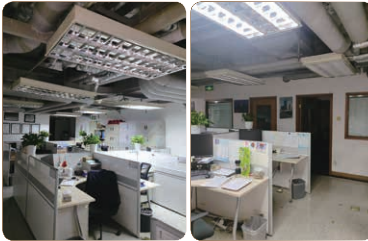
Inspections of office electrical equipment during non-standard working hours 非標時間辦公室關閉用電設備檢查
