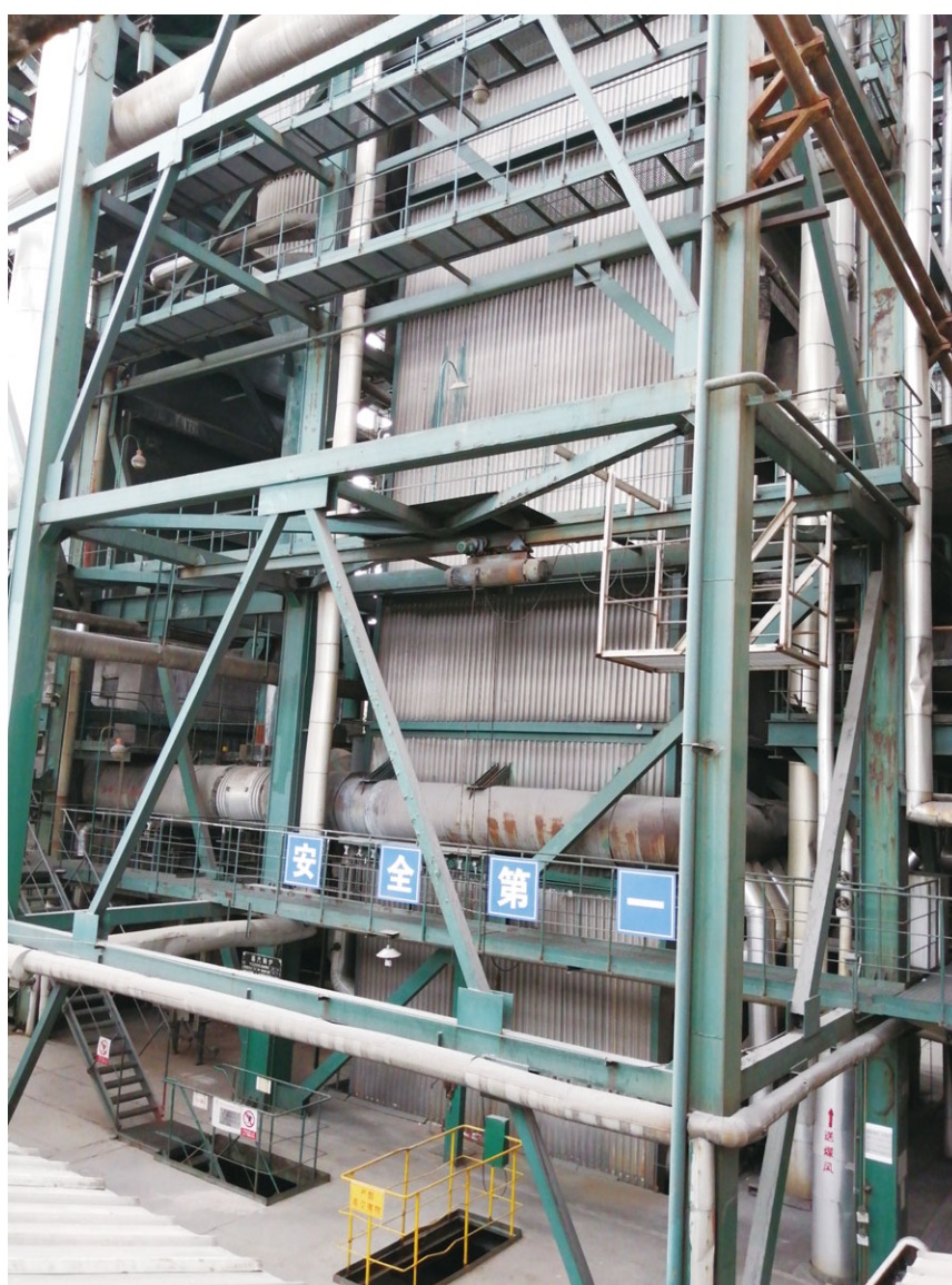
Circulating Fluidised Bed Boilers 循環流化床鍋爐
