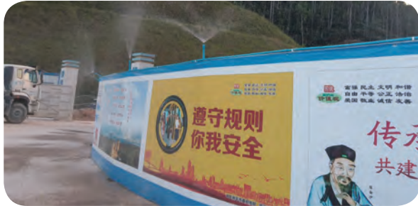
Automatic spray system with wall block 圍擋自動噴淋系統
