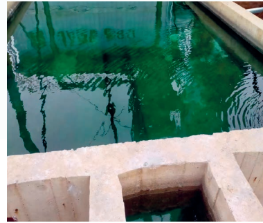
大連美食廠鍋爐軟化水處理 Boiler softened water treatment in Dalian food factory
