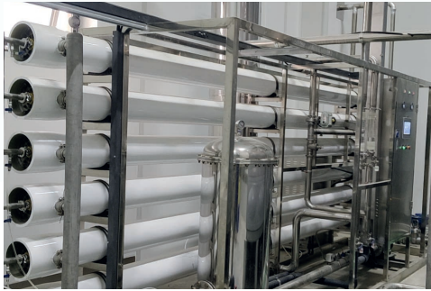
蚌埠鮮食廠反滲透處理設備 Reverse osmosis treatment equipment in Bengbu fresh food factory
