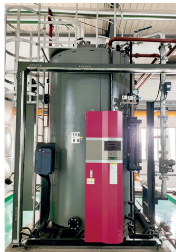
蚌埠新建飼料項目先進鍋爐 Advanced boiler in the new Bengbu feed project
