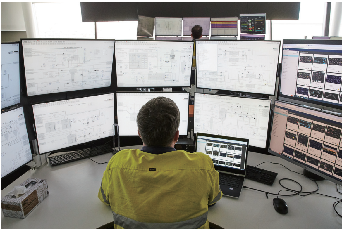
TLK奎納納工廠項目中控室 Control Room of the TLK Kwinana Plant Project
